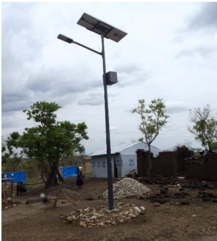
A lamp post installed by Oxfam in Uganda. Photo: Brian Reed
